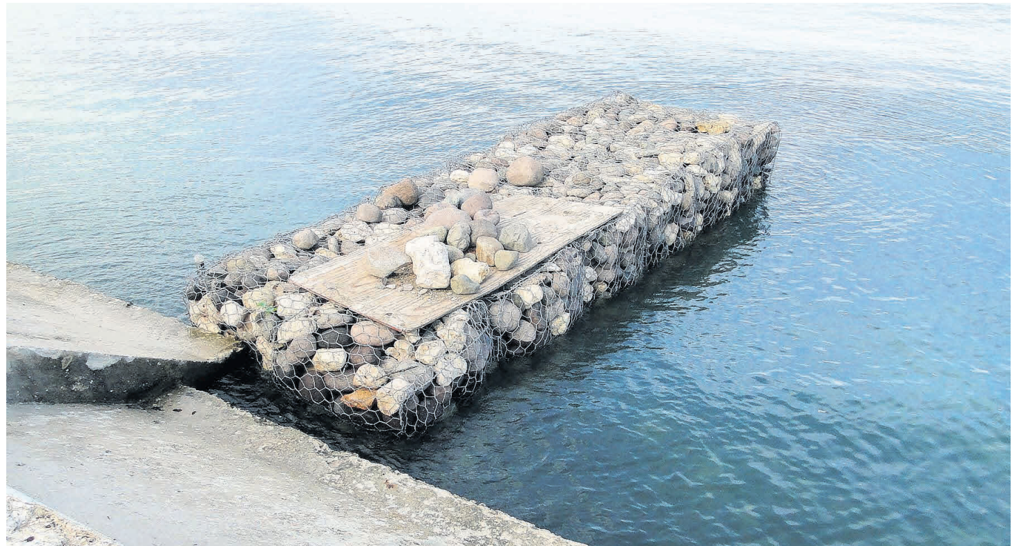
One of the newly constructed groynes in the vicinity of 'Dead End' Beach in Montego Bay.
