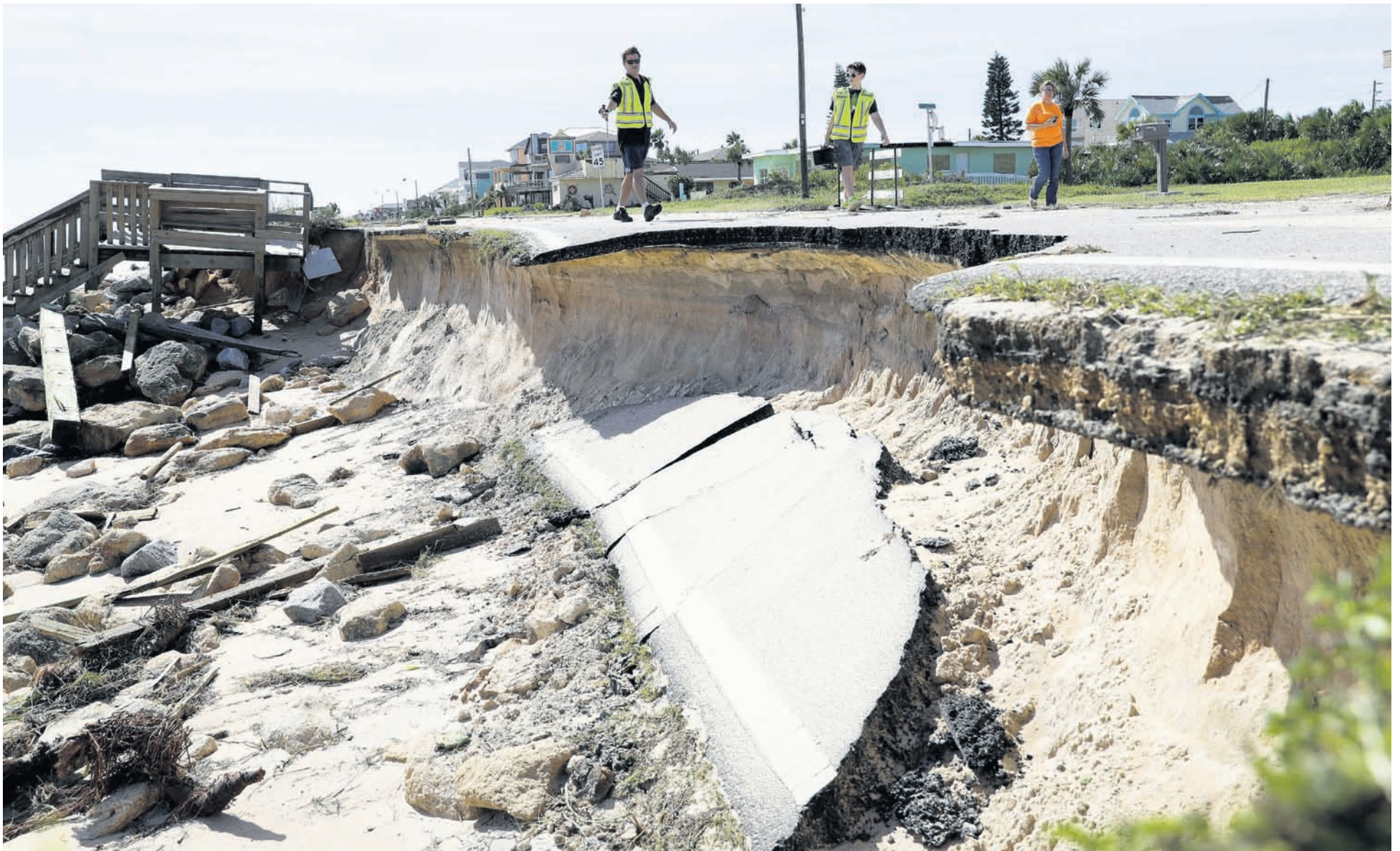
Officials photograph sections of highway A1A that were washed away by Hurricane Matthew, Saturday, October 8, 2016, in Flagler Beach, Florida. The damage from Matthew caused beach erosion, washed out some roads and knocked out power for more than one million customers in several coastal counties. AP
