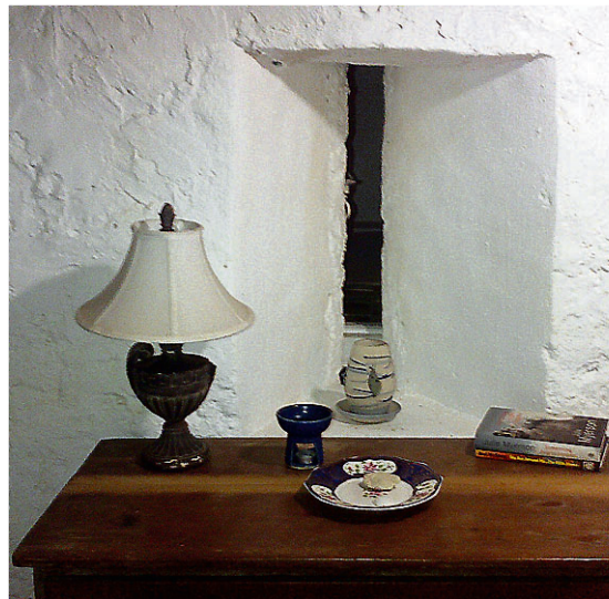
A gun slit in the basement of the Bromley Great House in Walkers Wood, St Ann.
